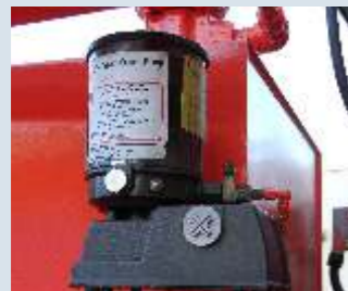
Centralized Auto greasing system for Pump
